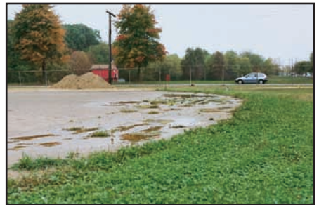
Poor skinned area drainage can leave a diamond in a muddy, unusable state. Most drainage problems result from poor design or bad maintenance practices.
