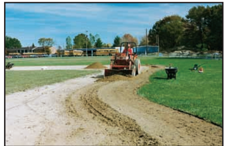
Once the sod has been removed, lower the grade to allow for positive surface drainage.
