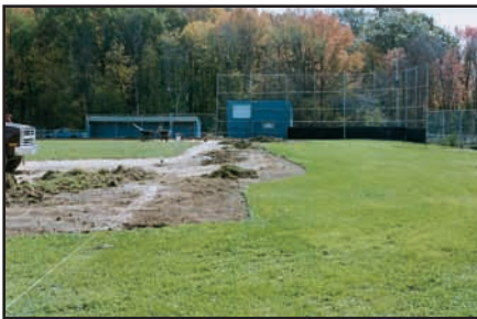
After the season, take time to cut away any lip that has formed at the edge of the grass. A standard sod cutter makes short work of the job.
